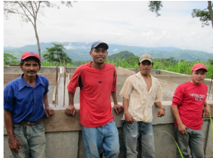
The tank for the irrigation system is in the final construction stages.
