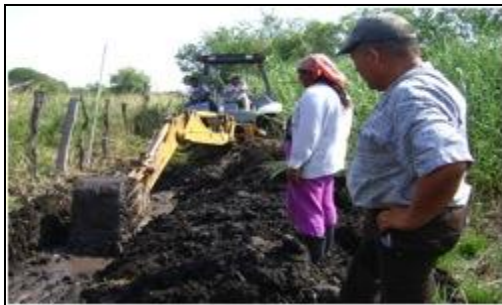
A new drainage system and irrigation canal were constructed during the quarter.
